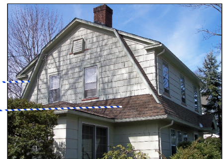
This roof, which is structurally a gable, appears to be a gambrel roof.
